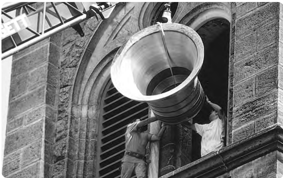
Bell number six cracked and was replaced in 1997 during the Archabbey Church renovation.
